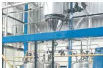
Stainless Steel Reactors
